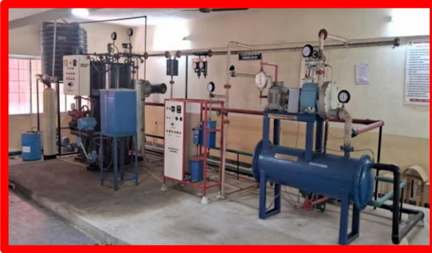
Thermal Engineering Laboratory
